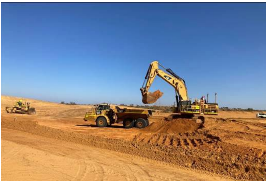
Figure 3 Excavation Activity at Ambassador North Pit, December 2021. This represents the substantial commencement of on-site works at the Mulga Rock Project.
